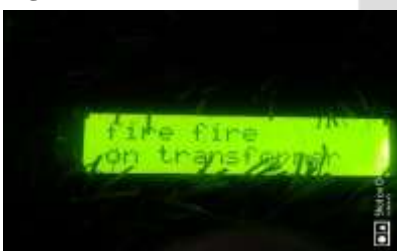
Figure 9: Fire on Transformer Detection
