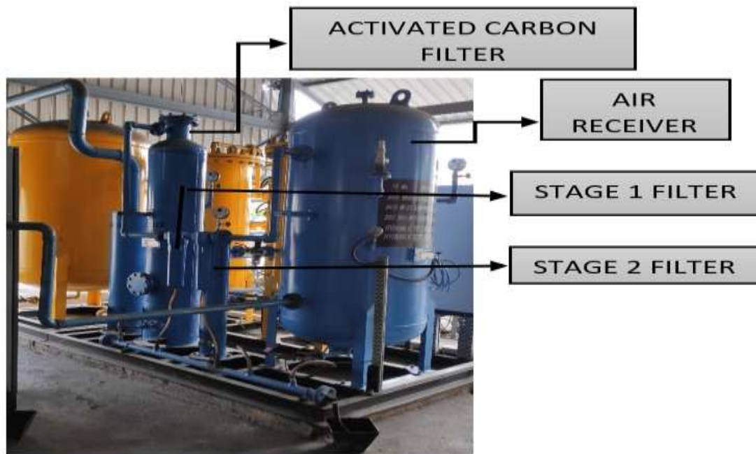
Figure 5: - Filters & Air receivers
