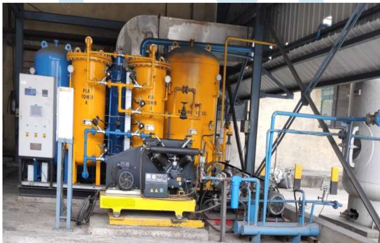
Figure 6: - PSA Nitrogen gas plant
