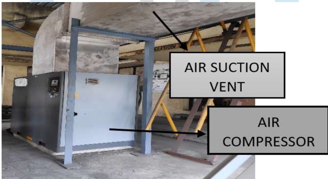
Figure 4: - Air suction vent & compressor
