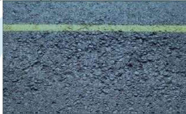
Figure 20. Segregation of Coarse Aggregate
