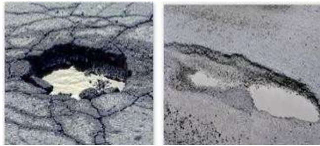
Figure 15. Pot Holes on road
