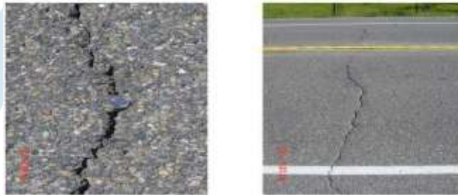
Figure 8. Transverse cracking on road
