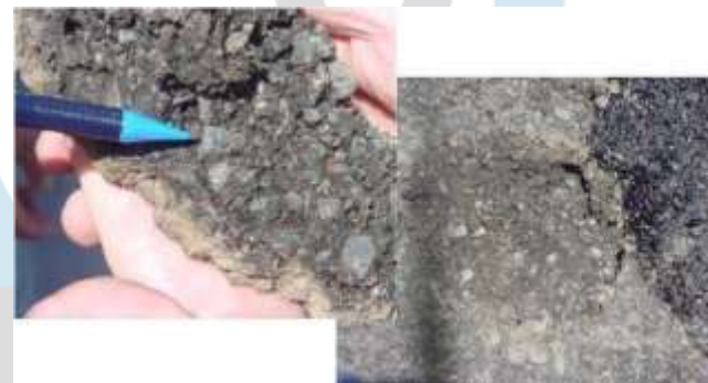
Figure 17. Stripping on road
