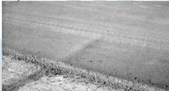
Figure 13. Overlay bumps on road
