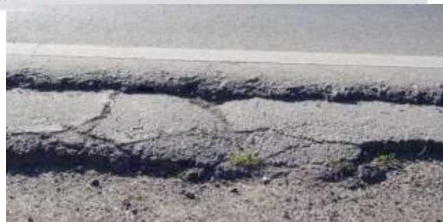
Figure 6. Edge cracking on road
