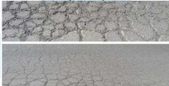
Figure 4. Fatigue cracking on road
