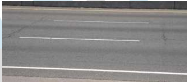
Figure 9. Reflections cracking on road
