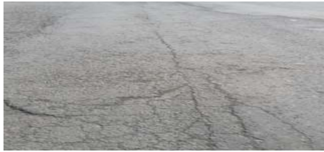
Figure 3. Longitudinal cracking on road
