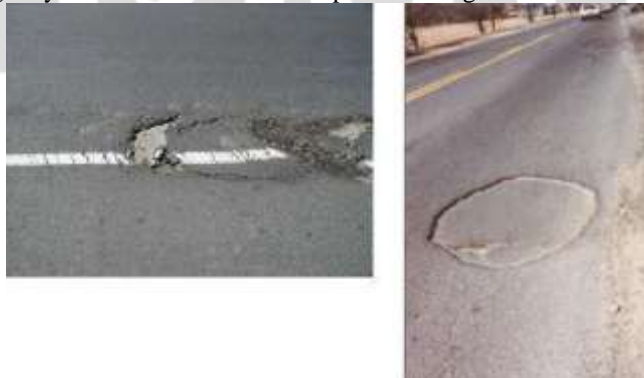
Figure 14. Delamination on road
