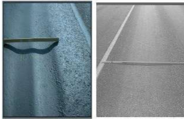
Figure 7. Rutting on road
