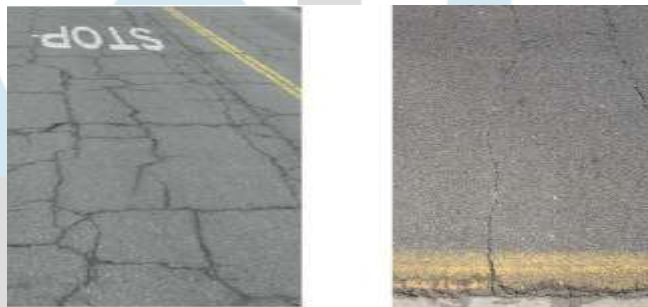
Figure 5. Block cracking on road
