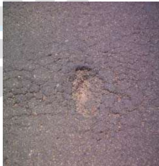
Fig : Pothole and Alligator Cracks
