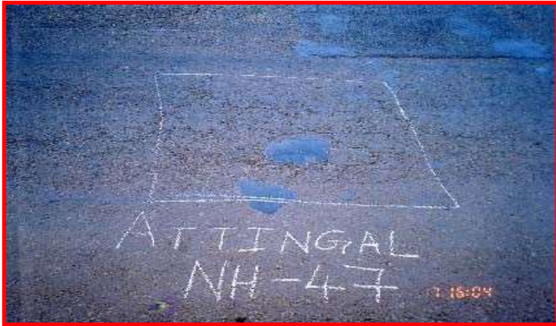
Fig : Cracks with patching
