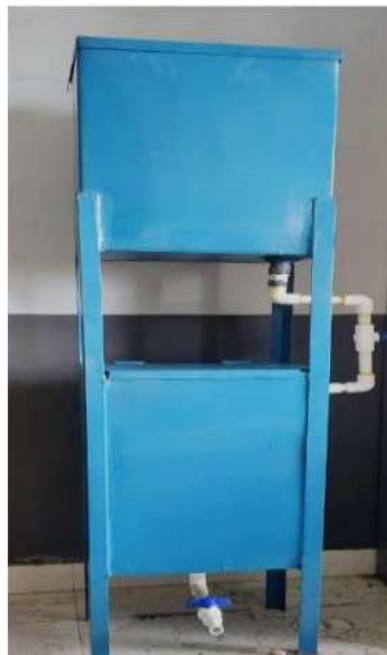
Fig:Coagulant Feeding tank cum filter
