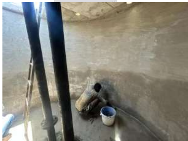
Fig. No.2- Detection of cracks formed in the bottom slab and walls of water tank
