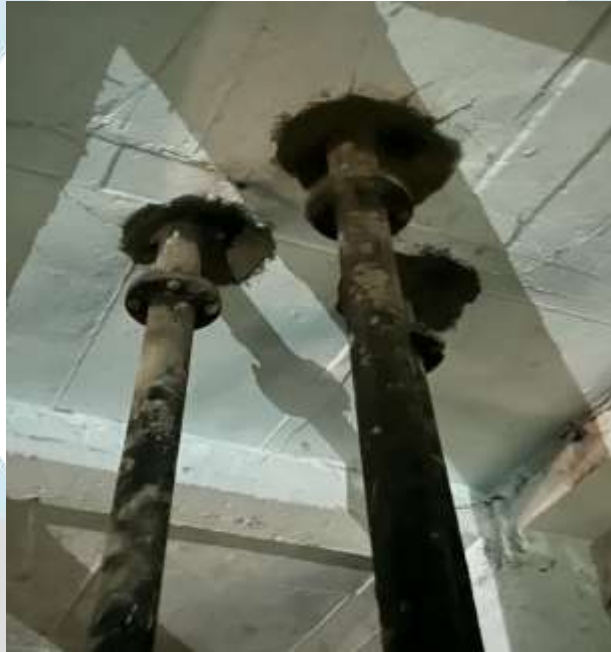
Fig.No.3- Cracks formed at bottom bottom slab, walls and joint between them are filled with
