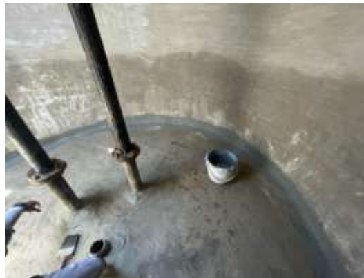
Fig. No.4 - Holes drilled in the slab for pipes are filled with chemically treated mortar
